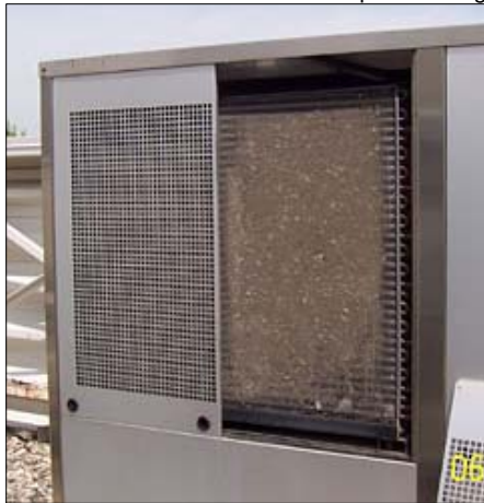
Severely fouled air cooled condenser (Provided by Air Solution Company)
